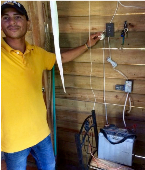
Picture 6: Solar Power System Ex. 1
