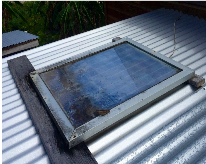
Picture 7: Solar Power System Ex. 2
